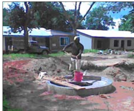
A Borehole driller finalizing his work at a COCOTO site in Songea.
